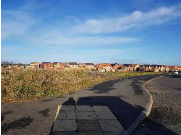
Figure 112 Housing currently being developed as part of the 'Roman Gate' development along the south side of the A46 west of Lincoln Road – located partly within the south side of the character area within the Lincoln 'edge'.
